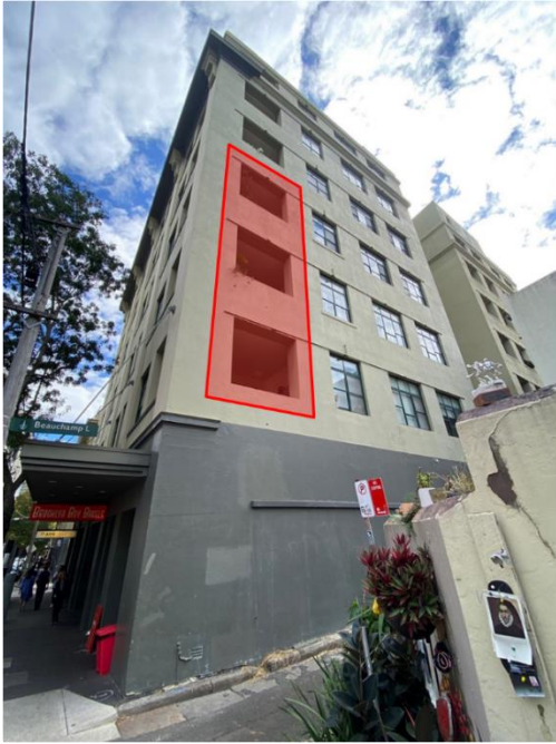
Figure 32: Balcony openings situated at Levels 1 to 3 on east elevation of 74-80 Reservoir Street impacted by the proposed development
